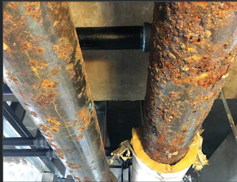
The image above shows extensive corrosion under the insulation.
